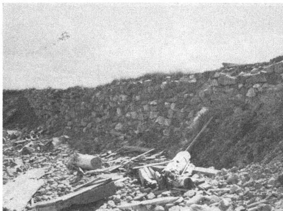
FIG. 14. Foundations of Royal Battery, Louisburg, revealed by heavy surf scour created by Hurricane Edna, 1954. Nova Scotia Research Foundation Photo.
