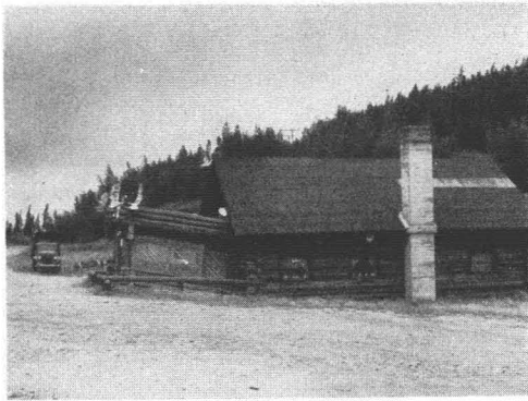
FIG. 1. A typical example showing what may happen if the builder is not familiar with the permafrost conditions: Bert and Mary's nice little inn at Richardson Highway between Fairbanks and Big Delta, Alaska, originally built with a veranda as a coffee-room. Ten months later, however, useful as a steep-sloping entrance only, to the settled main building. (Photo by the author August 24, 1955.)
