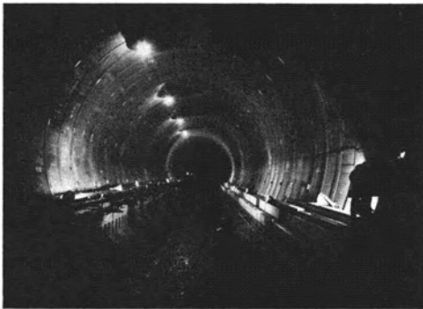
FIG. 8. A survey photograph of the length of the Second Mersey Tunnel which was subject to an experimental wriggle survey. Coordinates were determined on alternate rings (every 8 ft (2.44 m)). Points were observed on both premarked and natural surfaces. Concentric bull's eye targets and paint markings were used for premarking. The tunnel diameter was 31 ft 7 in (9.63 m).
