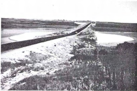
FIG. 13. A highway foundation failure in a saline lake basin where ground water is discharging and is creating a "quick" condition. The white patches beside the roadway are salt-saturated sediments pushed upward to the surface by foundation displacement and exposed by evaporation.
